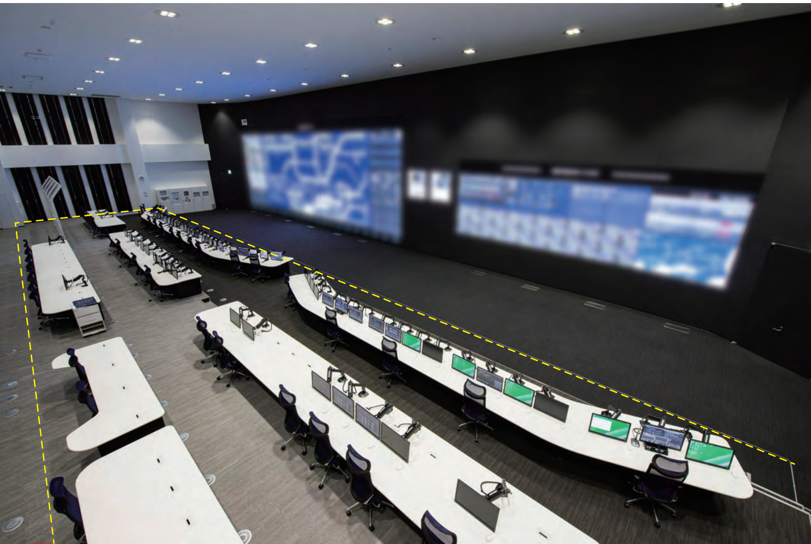
Traffic control center (281 m 2 surface)
