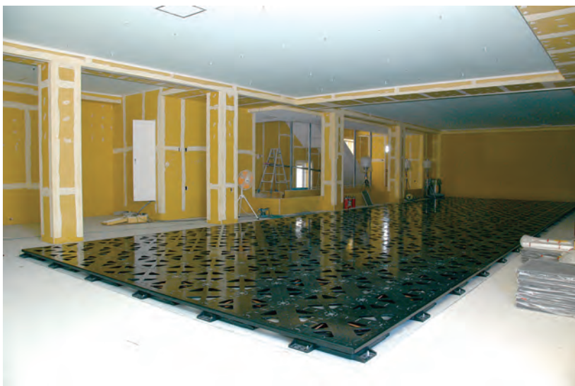
Installation of Seismic Isolation Module Model TGS
