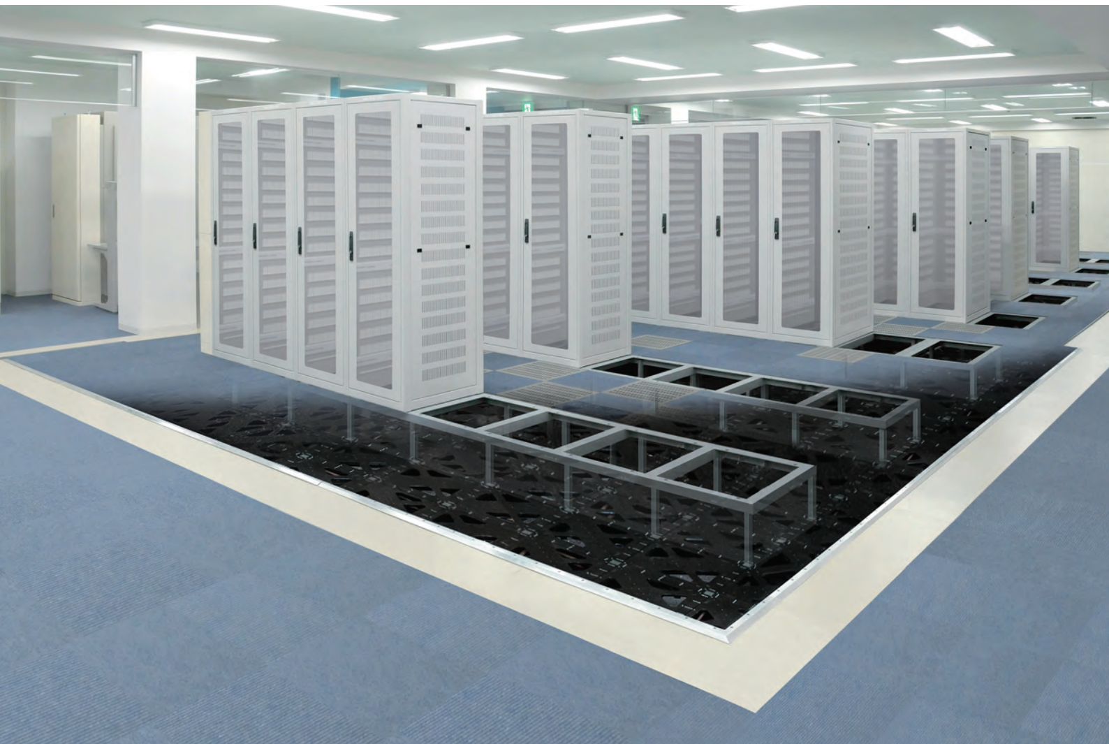
Toyohashi Cable Network inc: Data center
